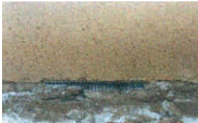
Fold wire mesh and place in holes in the foundation of houses
