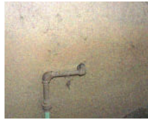
Look for gaps around pipes outside your home
